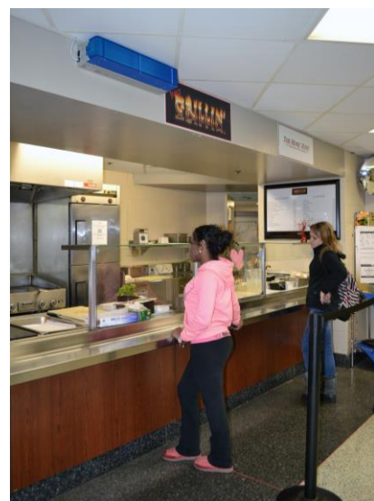
A GLO Upper-Room fixture disinfects the air above the cafeteria.
